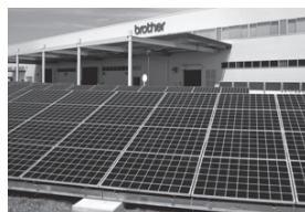
Solar panels aligned at the Kariya Factory
